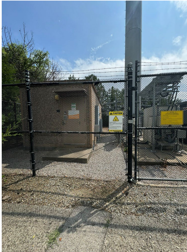
Exhibit 2: Photo of wireless communications facility and the eastern AT&T building and leasing area. Proposed generator will sit behind (south of) the building.
